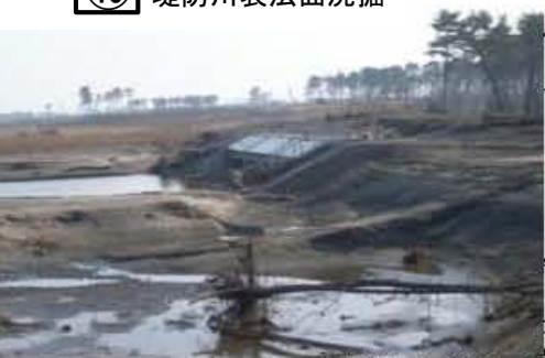
堤防川表法面洗掘
