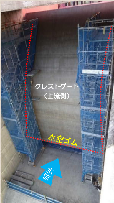
▲ View from the upstream side of the crest gate. The work site is high and sloped, so you can only see with your hands sweating...
