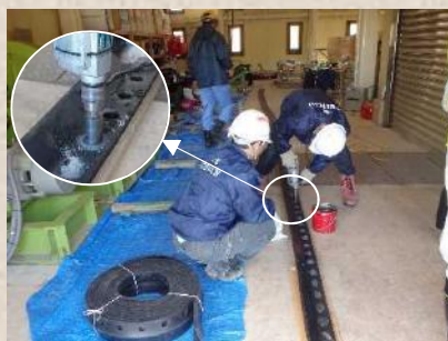
▲ Drilling holes into the long water seal rubber. Concentration is key to avoid failure!
