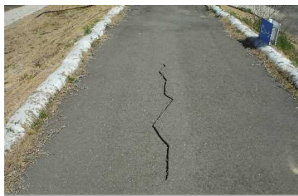
堤防天端の亀裂
