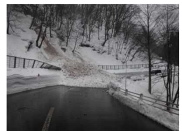
▲雪崩被災 (H29.2.17)
